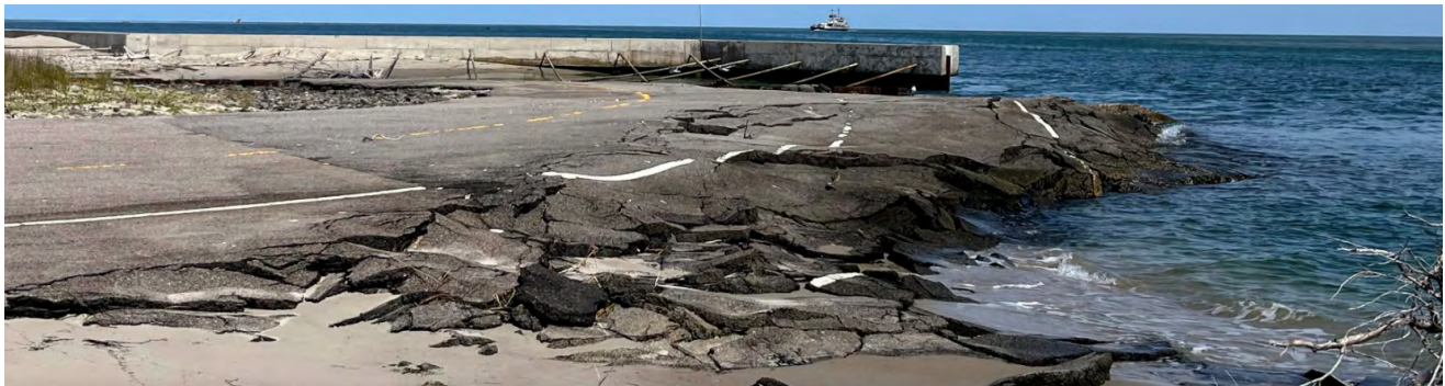
In 2019, South Dock's vehicle stacking lanes were lost to severe erosion (photo courtesy of the News & Observer)
